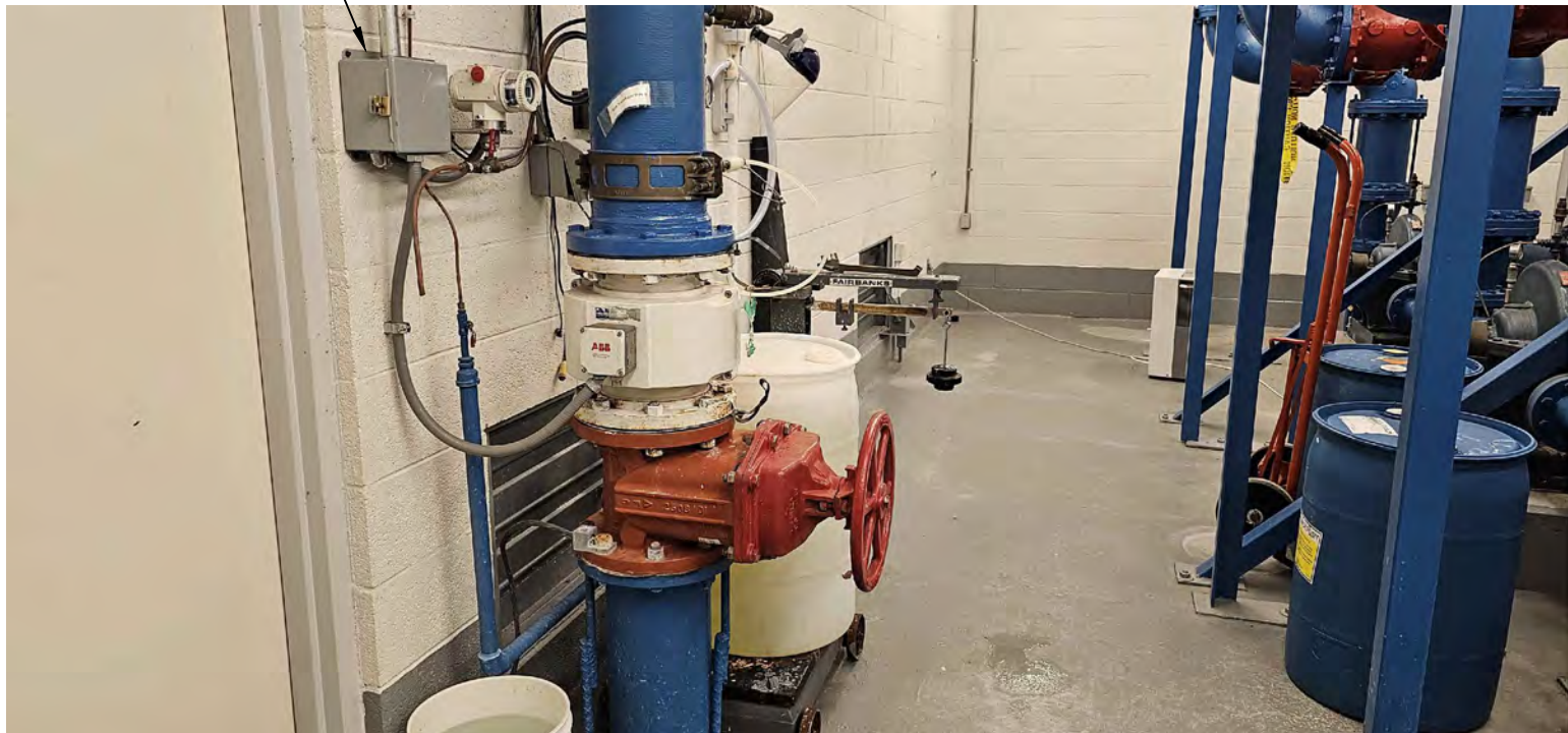
EXISTING BOOSTER STATION #2 INTERIOR
